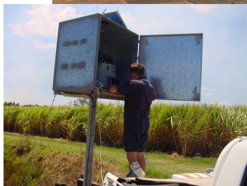
Plate 2.11 Strange's Drain (Site 6) galvanised box to house loggers, and solar panel
